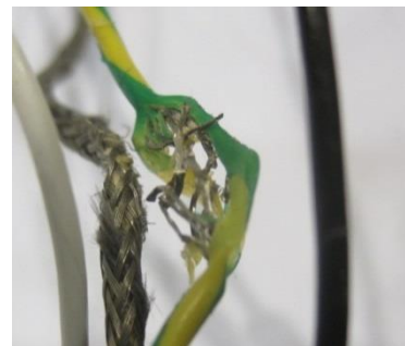
Figure 97: Defective earthing cable
