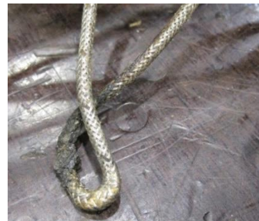
Figure 94: Squeezed heater cable
