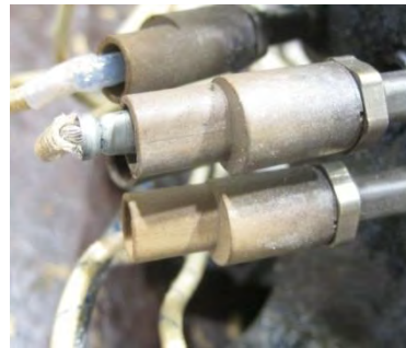
Figure 96: Torn-off heater cables, too small a bending radius
