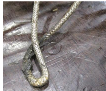
Figure 94: Squeezed heater cable
