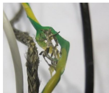
Figure 97: Defective earthing cable
